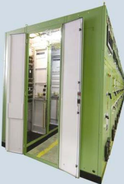
Duplex Relay and Control Panel
