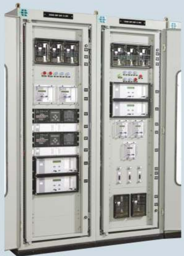
Generator Control Panel
